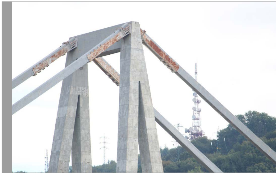
Corroding elements of the Morandi bridge before the collapse.
